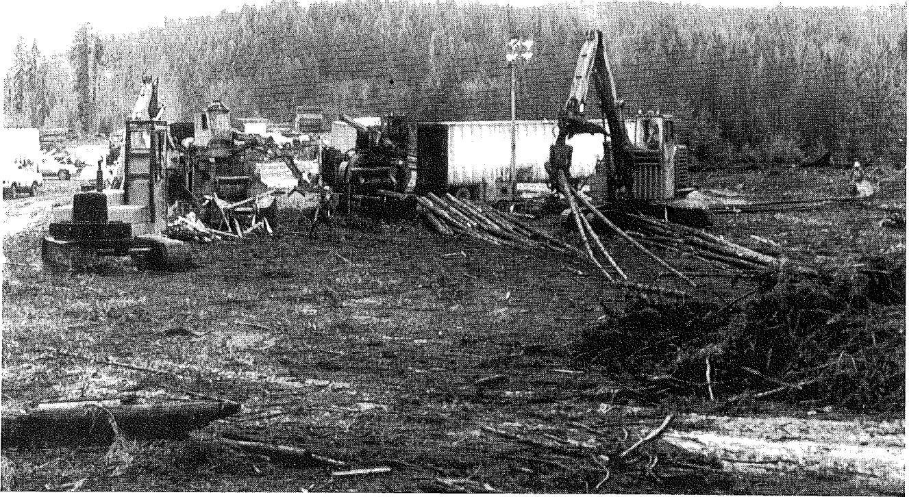
Specialisation and division - the landing for a high throughput chipping operation in Olympic Peninsula, Washington, U.S.A.
