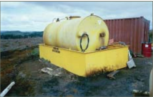
Self bunded fuel tank
