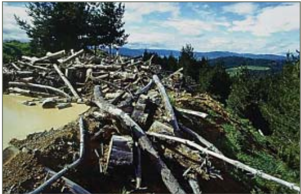
Water build up behind a 'birds nest' which could lead to collapse
