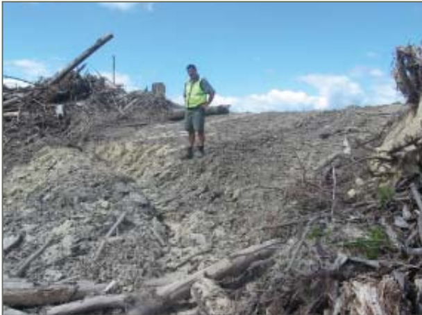
Drainage cut out, excavated to full width of track, discharging into logging slash.
