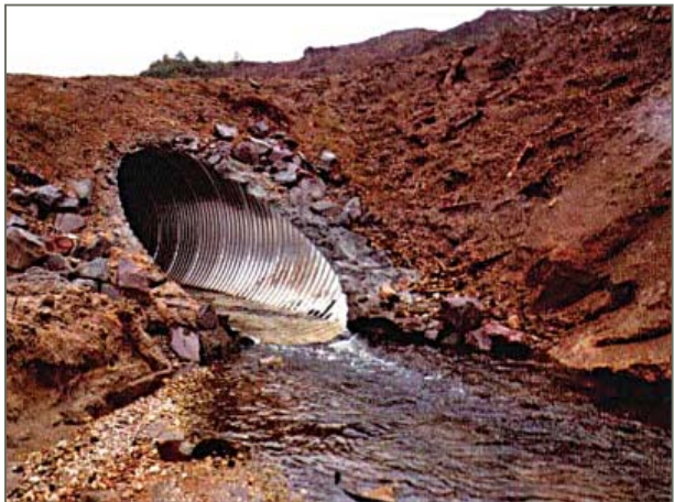
Single pipe culvert, with mitred outlet
