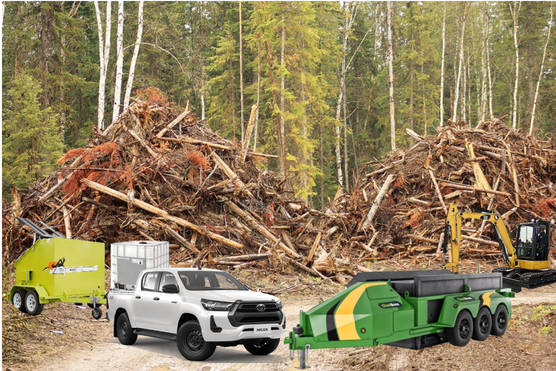
Figure 10. CharBoss operation supported by 1 x operator, 5.5T digger, 1000L water tote and a crew Ute with trailer
