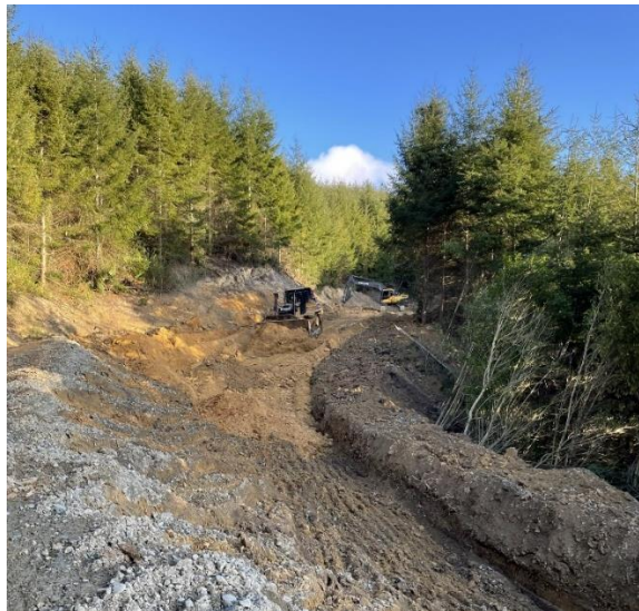
Figure 10: Undercut section of roading being reconstructed (Courtesy of Neil Thomas, Port Blakely).
