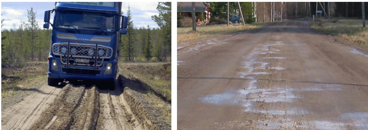
Figure 7: Unbound low volume roads exhibiting rutting (left) and pumping (right) (ROADEX Network, 2024).
