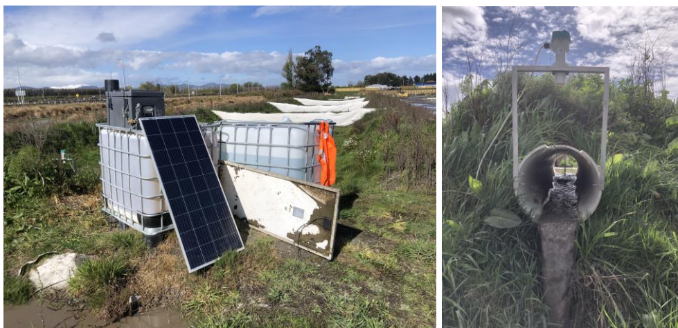
Figure 17: Flocculant 1000L IBC and onsite computer (left), Ultrasonic Sensor Set-up (right)
