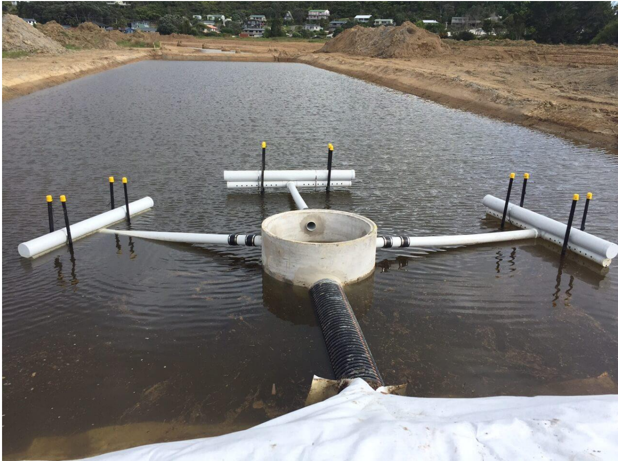
Figure 4: Floating Decant Arms within a Sediment Retention Basin (Cirtex Civil, 2024).
